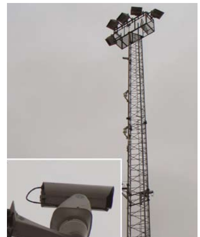
SR-100 installation at Copenhagen Airport
